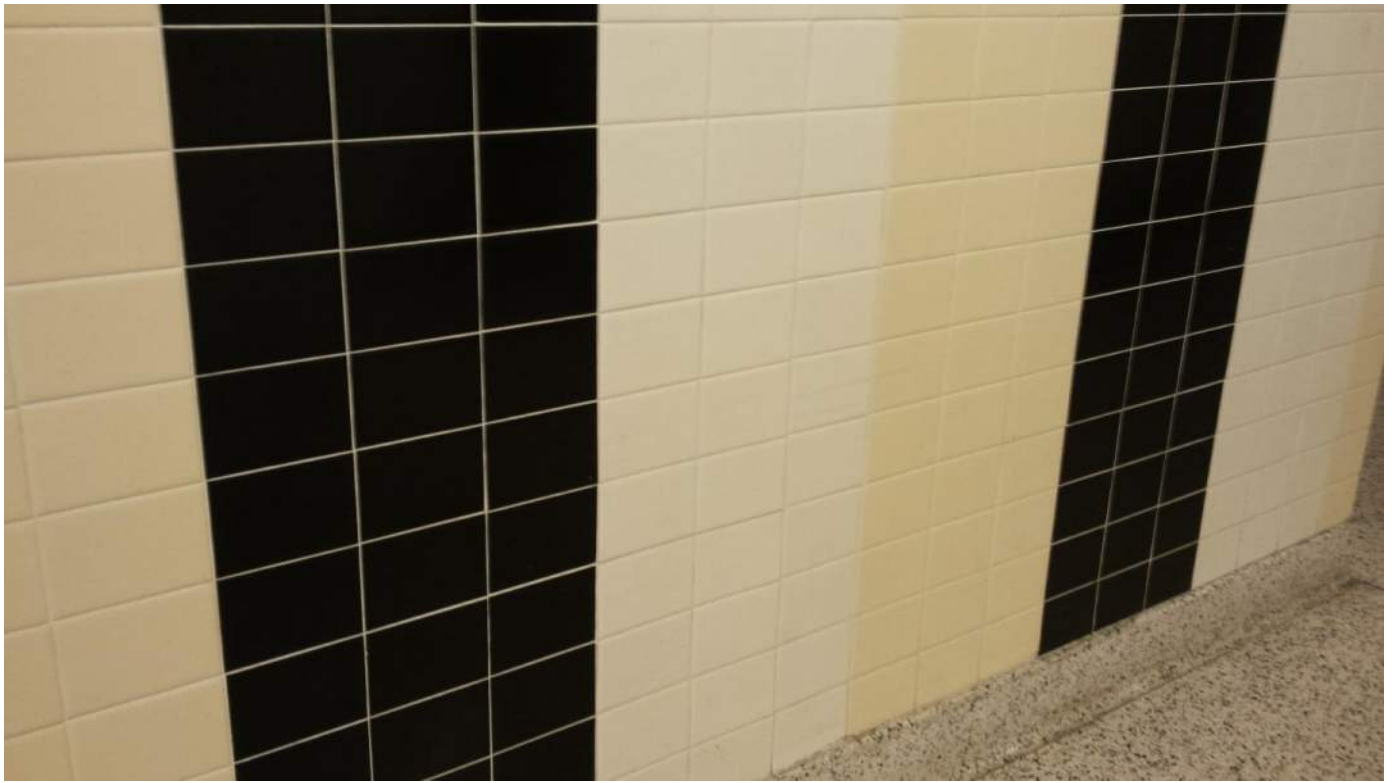
Photograph 3 – A view of the white, yellow, and black ceramic wall tiles that are positive for lead based paint.
