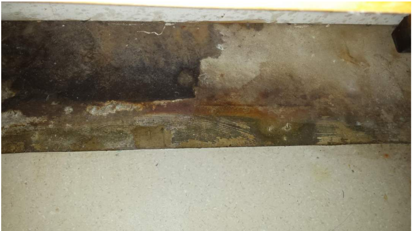
Photograph 6 – This photo shows the asbestos containing mastic beneath the beige vinyl floor tile (which also contains asbestos).
