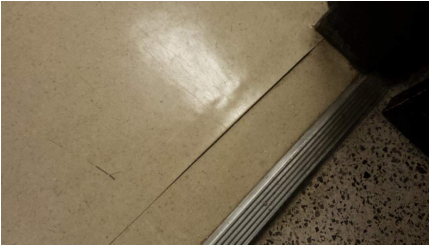
Photograph 5 – This photo shows the beige vinyl floor tile that contains asbestos.
