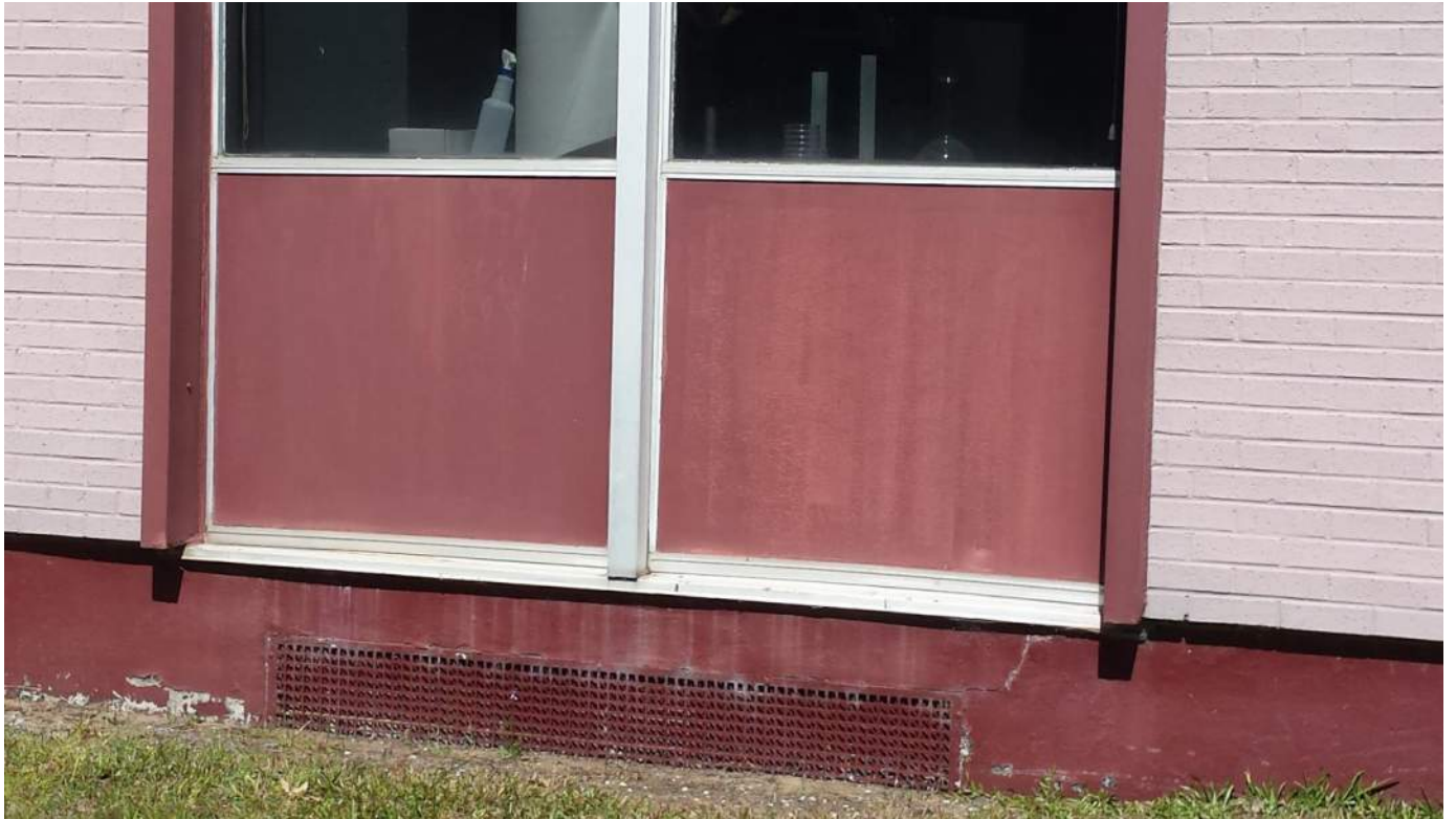
Photograph 4 – This photo shows the red, metal window panels that contain lead based paint.
