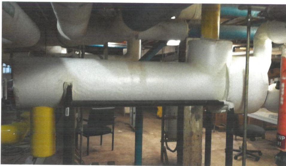
Two heating water distribution pumps (HWP-1 and HWP-2), of differing manufacturer, piped in parallel, circulate the heating water to the air handling unit heating coils.
