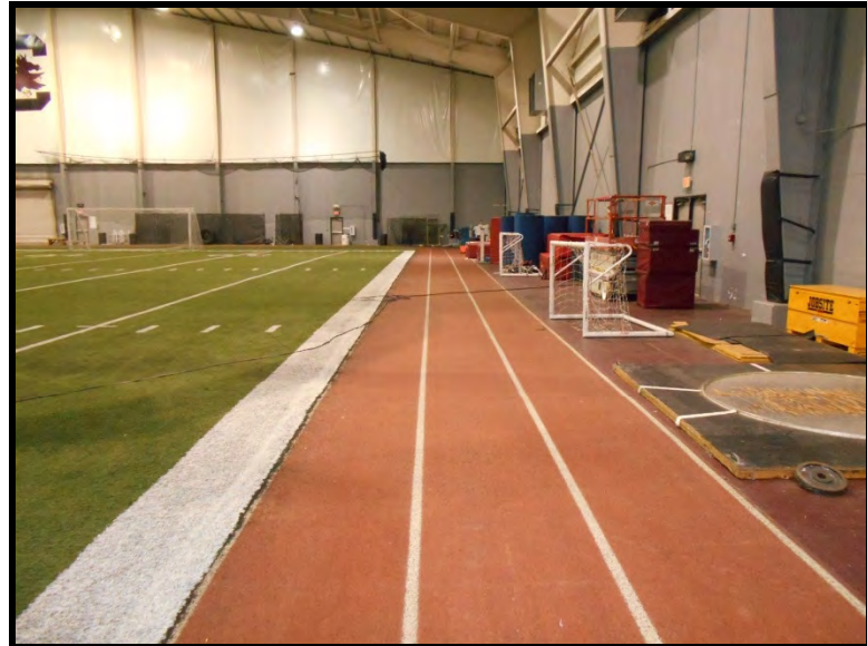
2 General view of mercury-containing track surface material (Approximately 7,550 sq. ft.).
