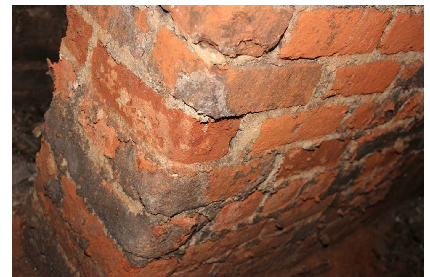
TYPICAL CONDITION OF MASONRY WALLS UNDER STAIRS
