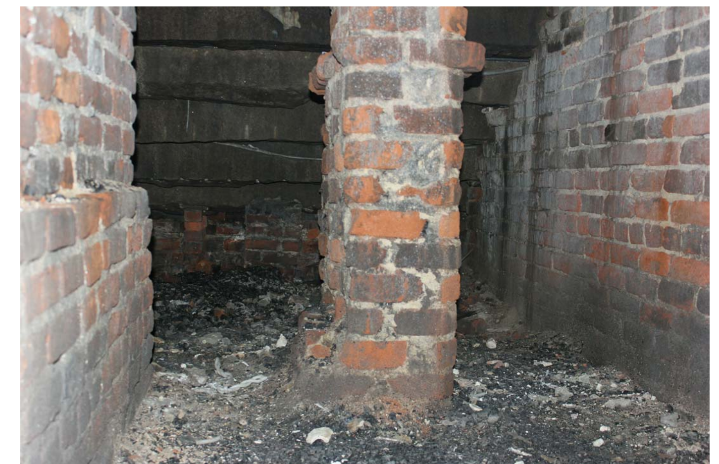
TYPICAL CONDITION OF MASONRY WALLS UNDER STAIRS
