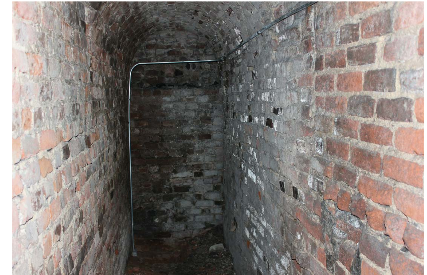
TYPICAL CONDITION OF MASONRY WALLS UNDER STAIRS
