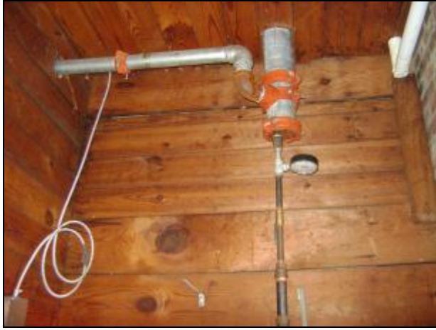
View of riser coming through ceiling
