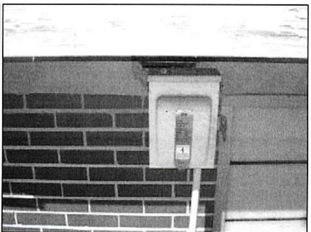
View of electrical disconnect
