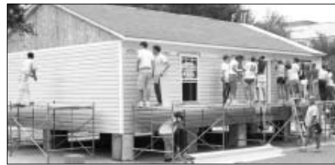
Students volunteered their time and construction skills to build a house for Habitat for Humanity.
