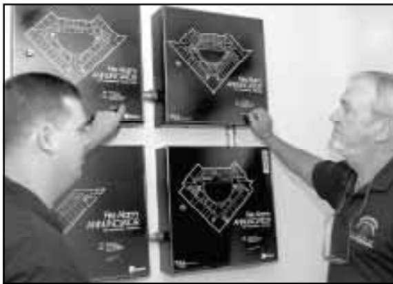
Campus Fire Marshal David Castine, right, and staff member Todd Griffin review the fire alarm system at Swearingen Engineering Center.
